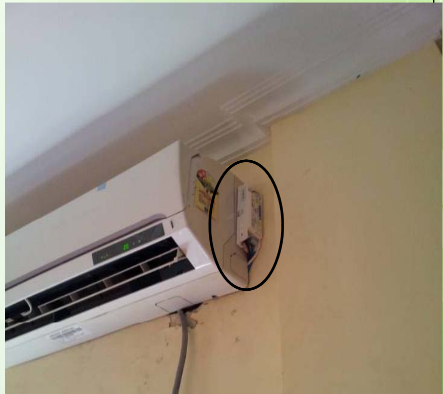
Split AC with AC Energy Controlling Unit
