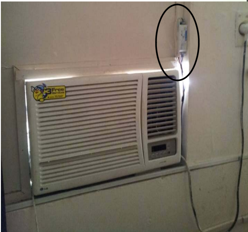
Window AC with AC Energy Controlling Unit
